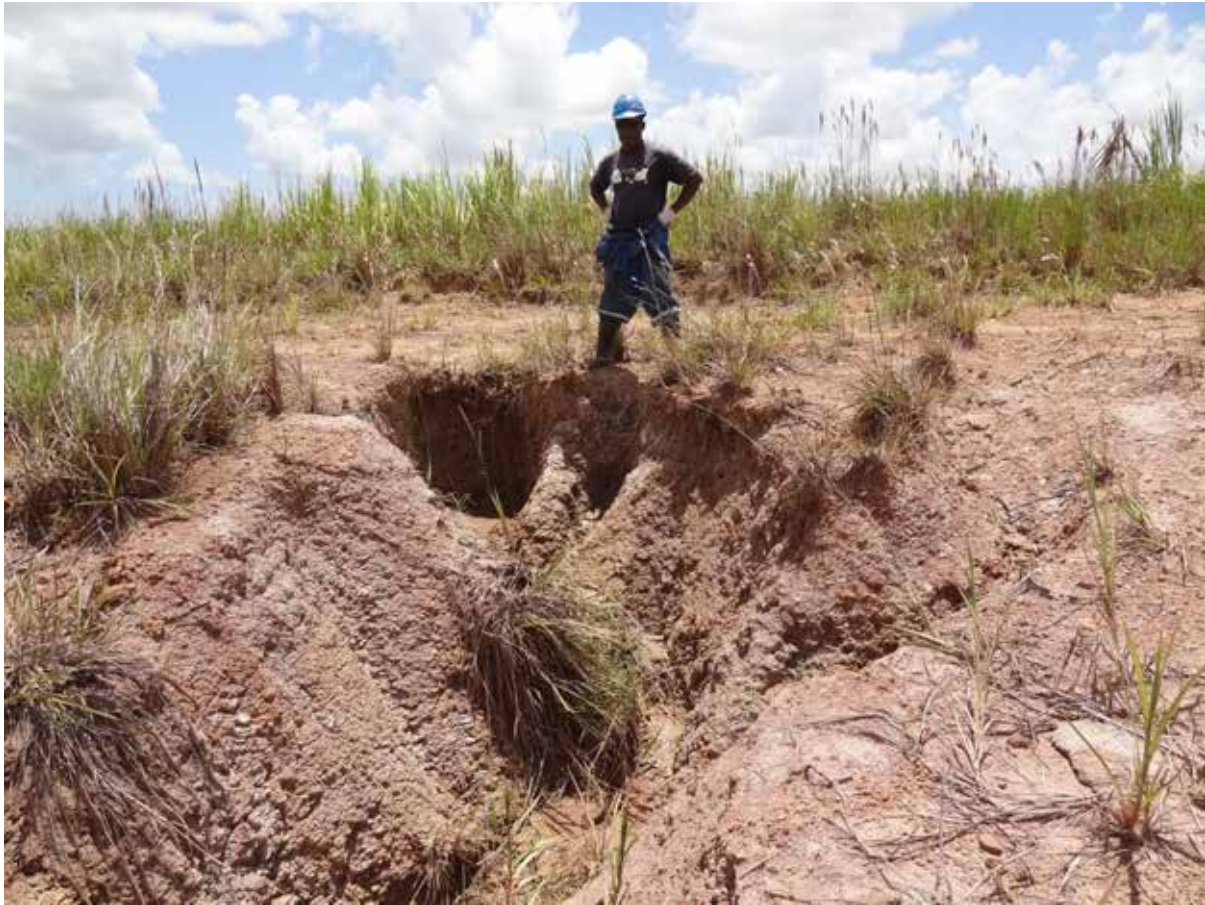
FIGURE 3.4 COUVA CHILDREN'S HOSPITAL, COUVA, TRINIDAD – EROSION CHANNEL CAUSED BY SURFACE FLOWS.
